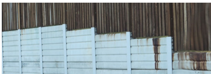
Photograph 1 - Unpainted hardwood causing tannin stains on concrete
