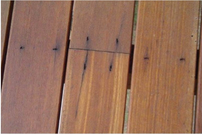
Photograph 3 - Iron staining due to ungalvanized nails (also nails are not appropriate type)
